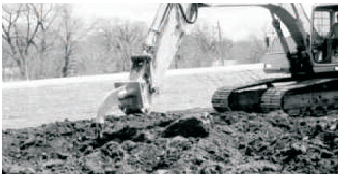
Figure 26: Scarifying the Soil - during construction significantly improves the chances of any vegetation establishment
