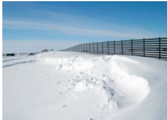
Figure 21: Structural Snow Fence
